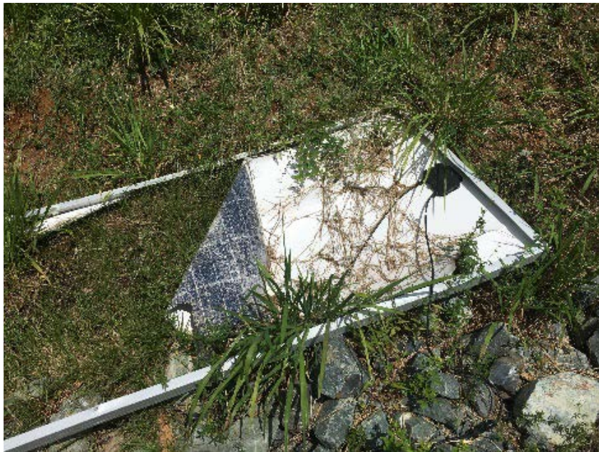
Figure 3. PV module torn from racking, lying face down, shows laminate failure
