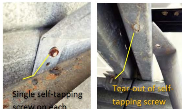
Figure 5. Examples of hardware failure
