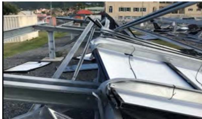
Figure 4. Examples of failure of clamp (top left of photo) causing attached modules to overturn
